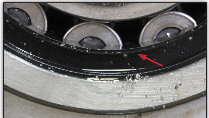
Metal flakes have pooled at the bottom of this bearing. It needs to be replaced.
